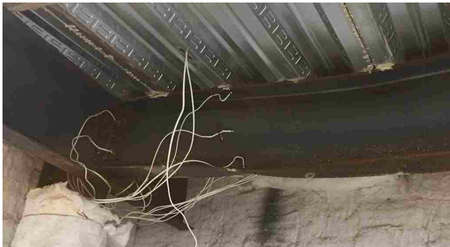
Figure 72 – Plastic Hinge in Unprotected Beam
