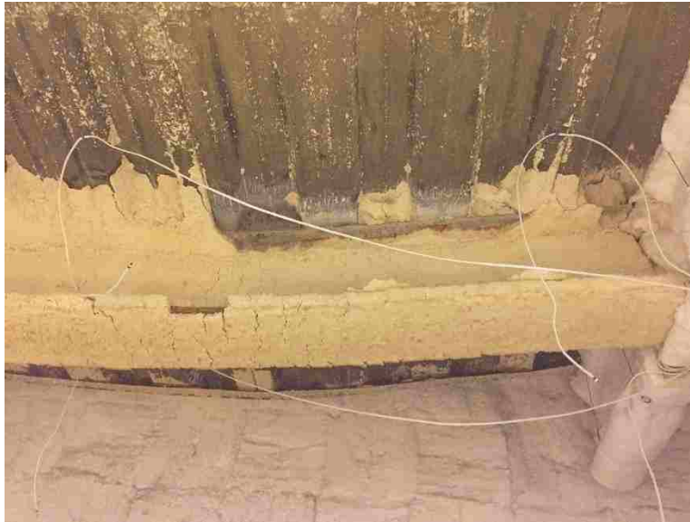
Figure 52 – SFRM chunks missing on flanges
