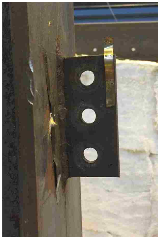
Figure 13 – Shear tab connection after the test
