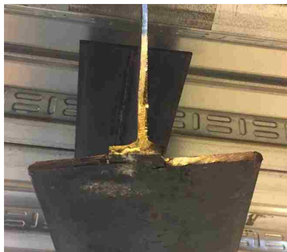
Figure 74 – Rupture in Web to Flange Connection
