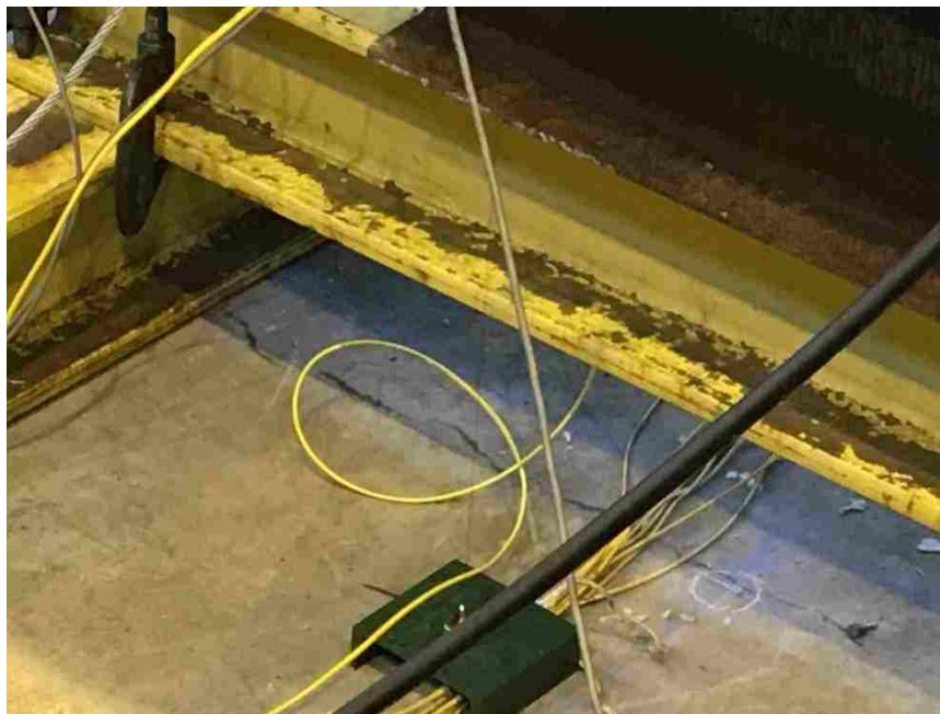
Figure 11 – Close up of longitudinal crack
