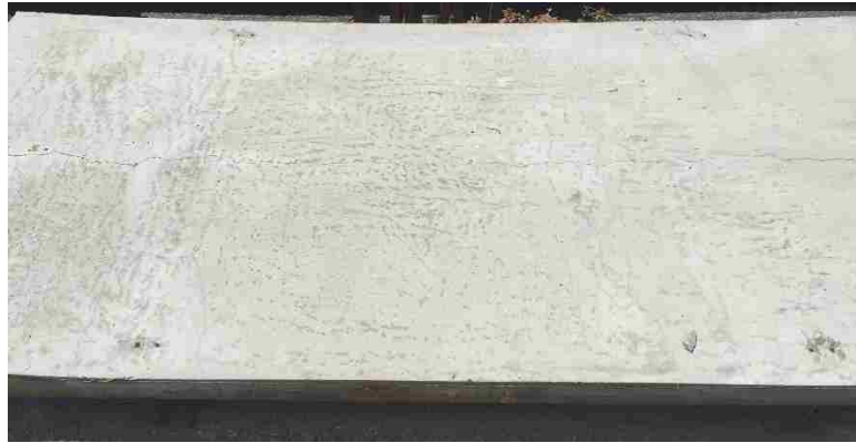
Figure 10 – Photo of top of slab after Test 1
